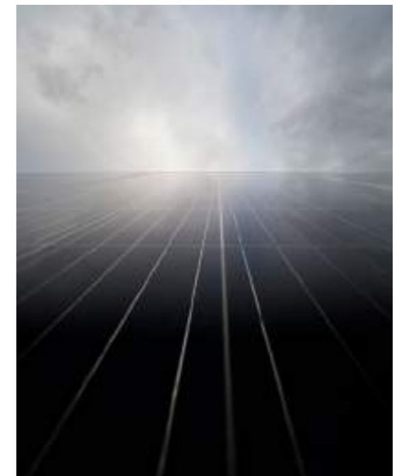
→ Photovoltaic installations at Cosentino
